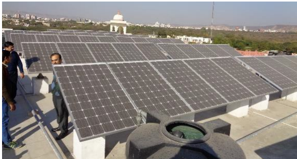
Figure 9: SPV system at the rooftop
